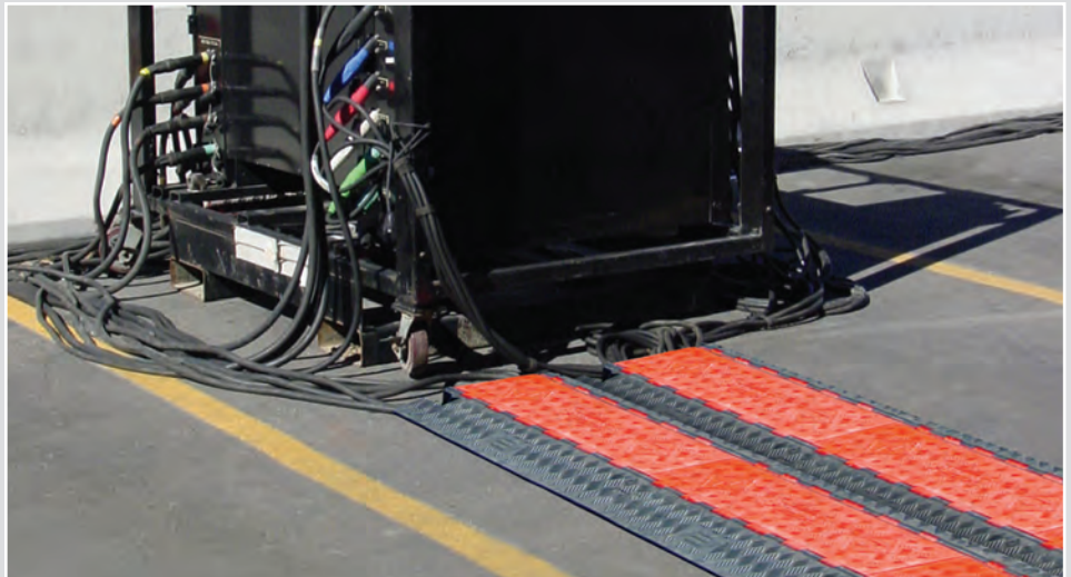
Guard Dogs in use with a power distribution box
