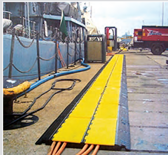
AMS in use at Naval dock yard
